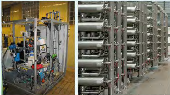
Figure 3: Left picture: Pilot installation of backwash process; right picture: current full-scale backwash water treatment by UF at WAG
